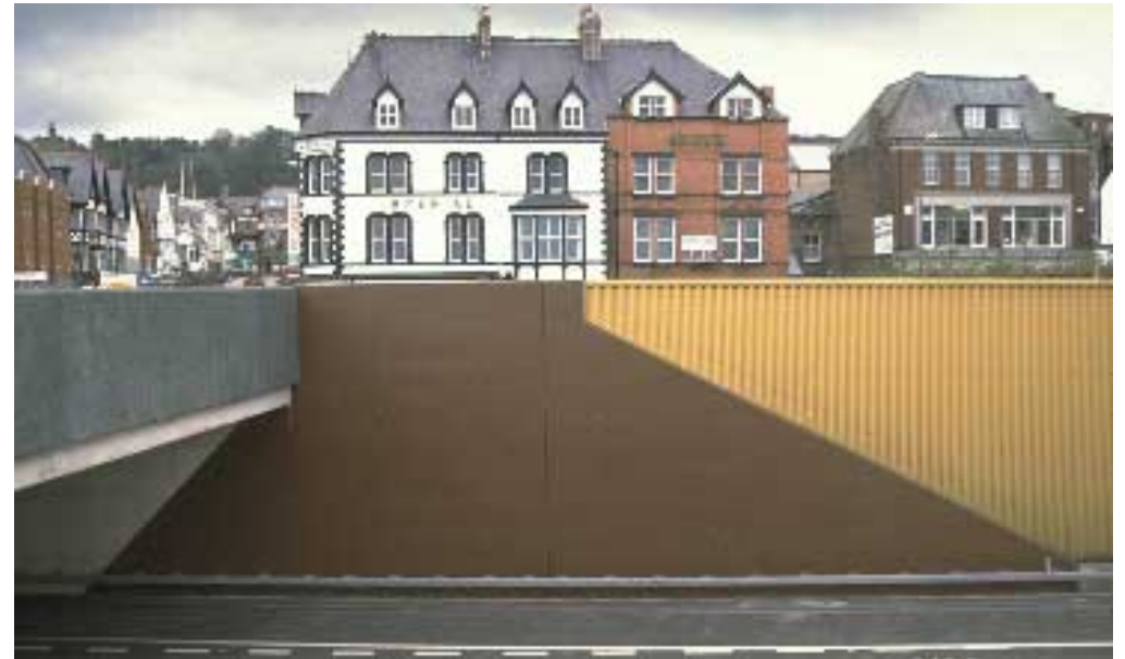
Colwyn Bay Concrete Wall This retaining wall has been raised to provide screening and separation for the adjacent public areas, where space does not permit other measures; and a separate barrier on top of the wall would degrade the design concept and cause maintenance problems
