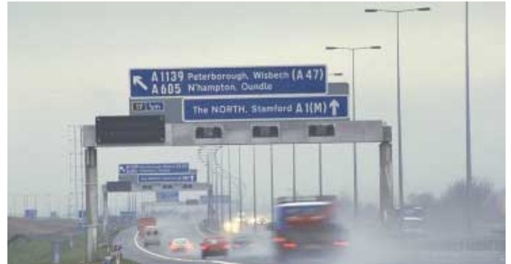
A1 (M) Gantries Network control projects: The structures, sometimes combined with their flashing message signs, can be extremely obtrusive. Cable-routes also need assessment to avoid damage to established vegetation and grassland habitats
